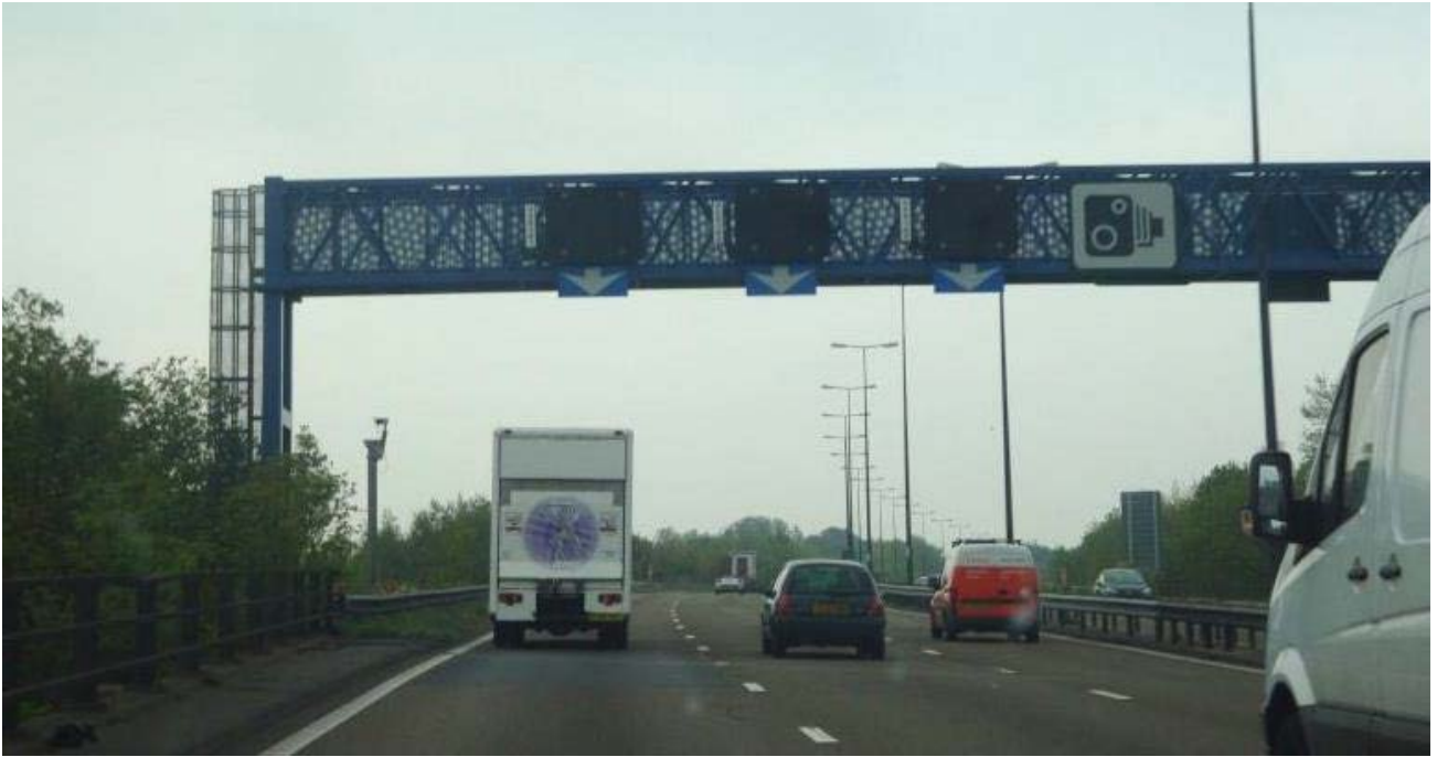
Figure 1 – Electronic signals on an overhead gantry
